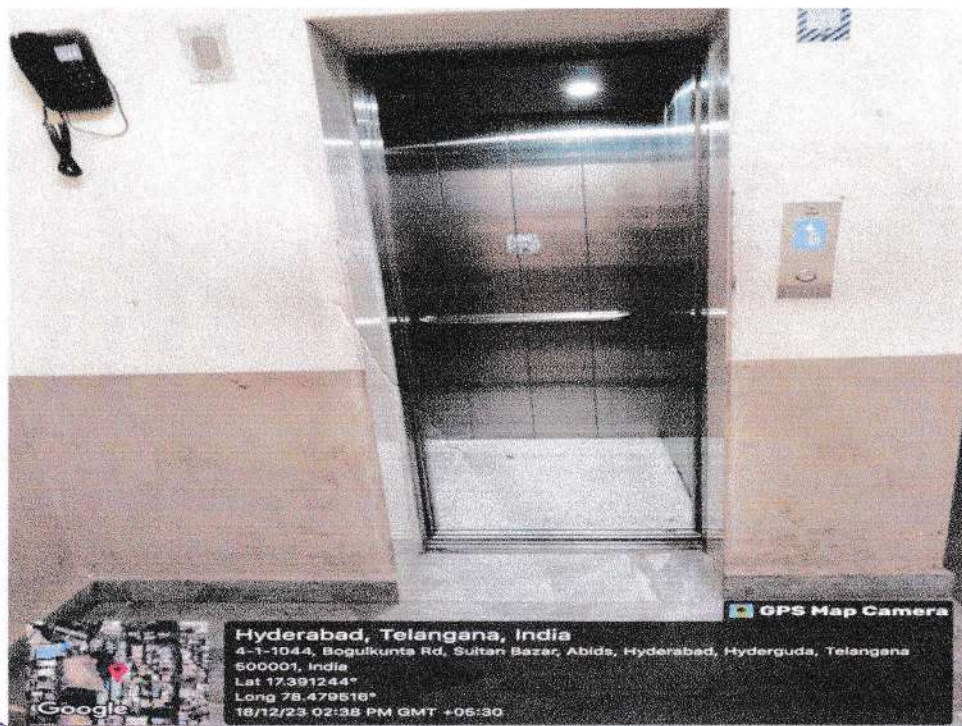
Lift in 'E' block
